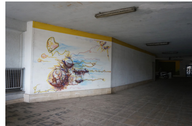
Figure 6.14. Graffiti on the wall of a dark passageway in PTS
